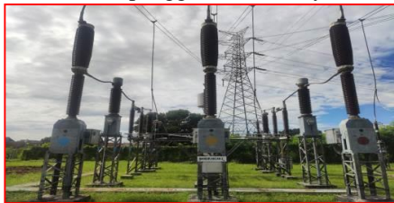
Gambar 3. PMT 150 kV Single Pole Mandirancan I
